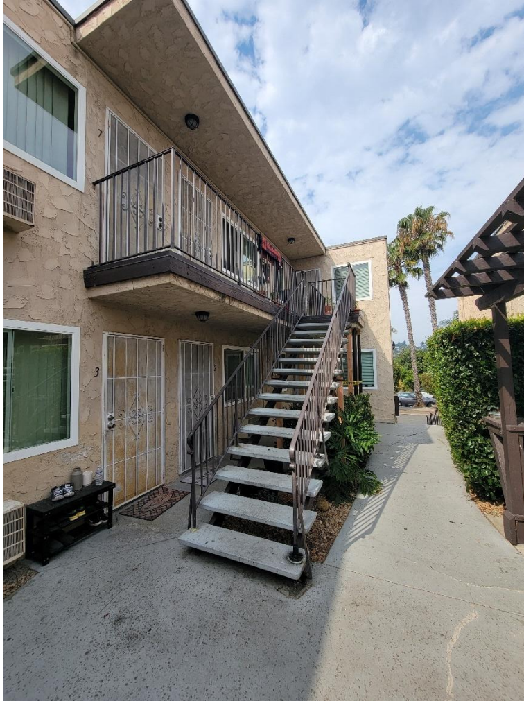
Picture 27: South stair at 4653 3 rd street which the right (west) stair railings is wobbly and unsafe.
