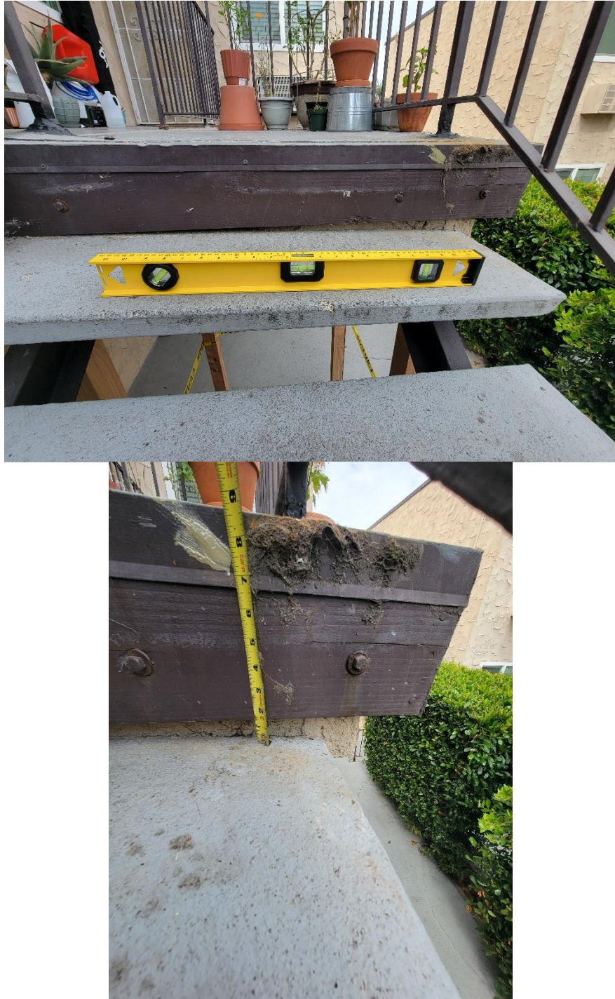
Picture 32: Stair is settled on the west side approximately 1"
