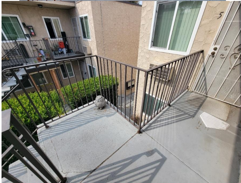
Picture 16: View of landing railing which is wobbly and unsafe
