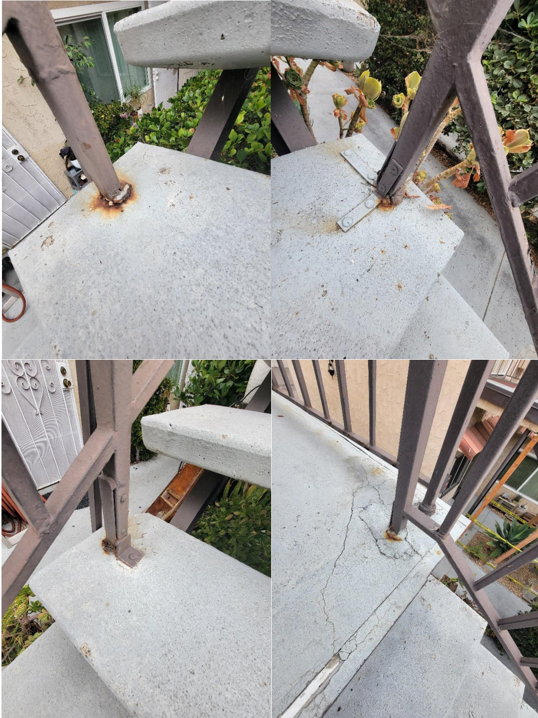
Picture 5: Non-standard post anchorage to the concrete treads or cracked concrete topping on landing.
