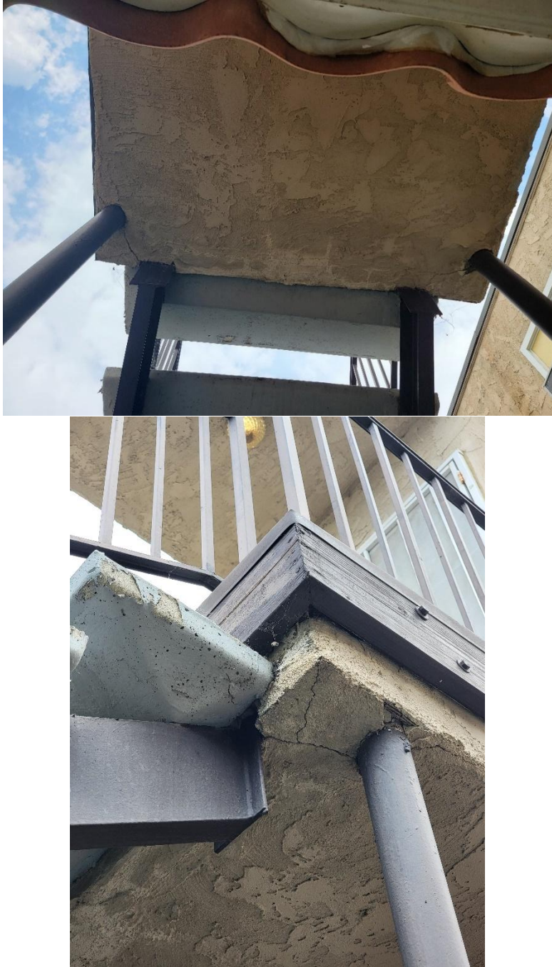
Picture 7: View of stair steel stringer connection to the landing's framing which is not exposed to be verified. Cracked stucco around the steel posts.
