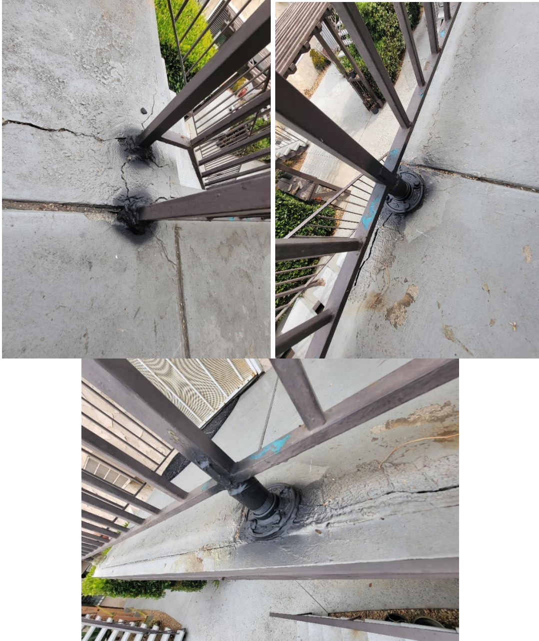
Picture 36: Different non-standard railing post anchorage to the landing's cracked concrete topping.
