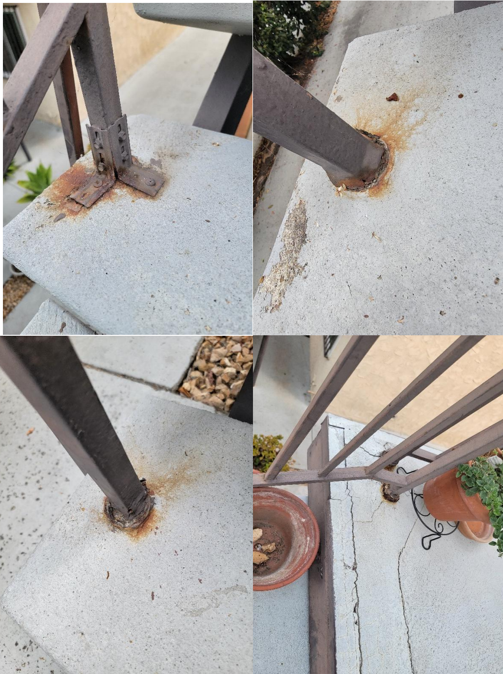
Picture 22: Different non-standard stair railing post anchorage to the concrete treads and railing landing to cracked concrete topping.
