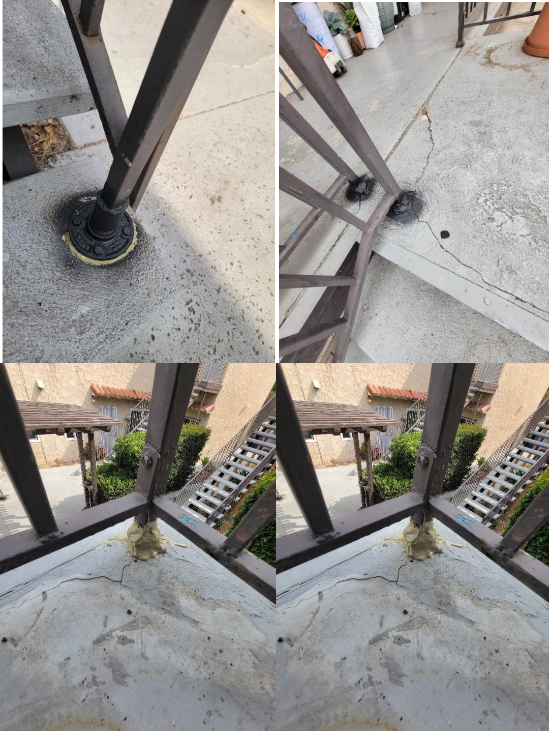
Picture 35: Different non-standard railing post anchorage to the landing's cracked concrete topping.
