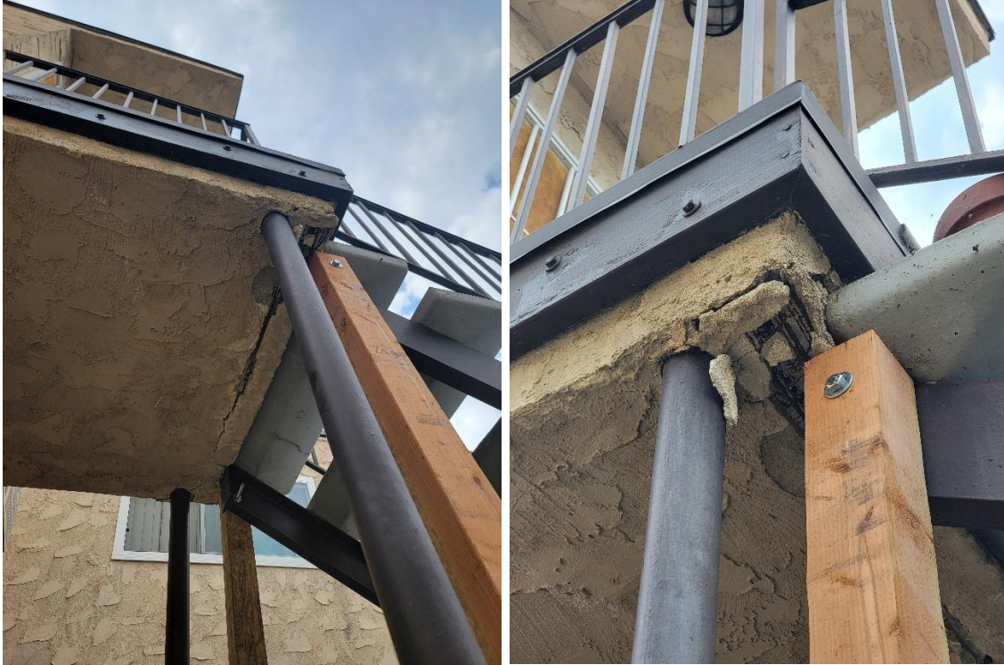
Picture 25: View of stair steel stringer connection to the landing's framing which is not exposed to be verified. Temporary shoring has been constructed. Cracked stucco along the stair connection observed.
