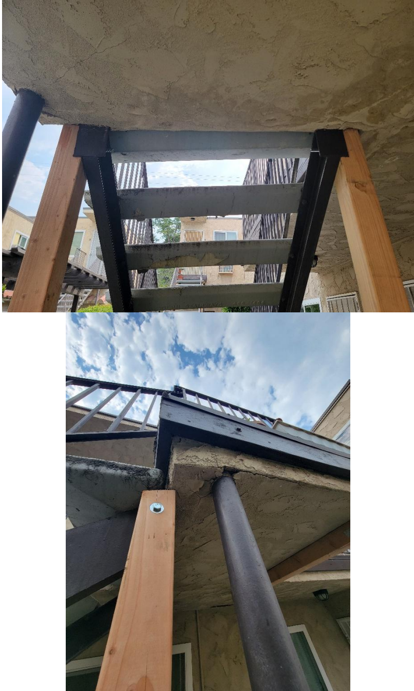
Picture 30: View of stair steel stringer connection to the landing's framing which is not exposed to be verified. Temporary shoring has been constructed. Cracked stucco along the stair connection observed.
