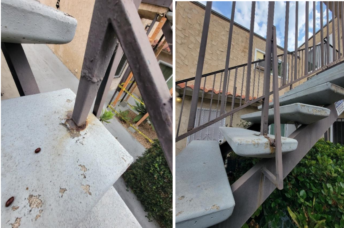
Picture 4: Different non-standard post anchorage to the concrete treads and steel stringer
