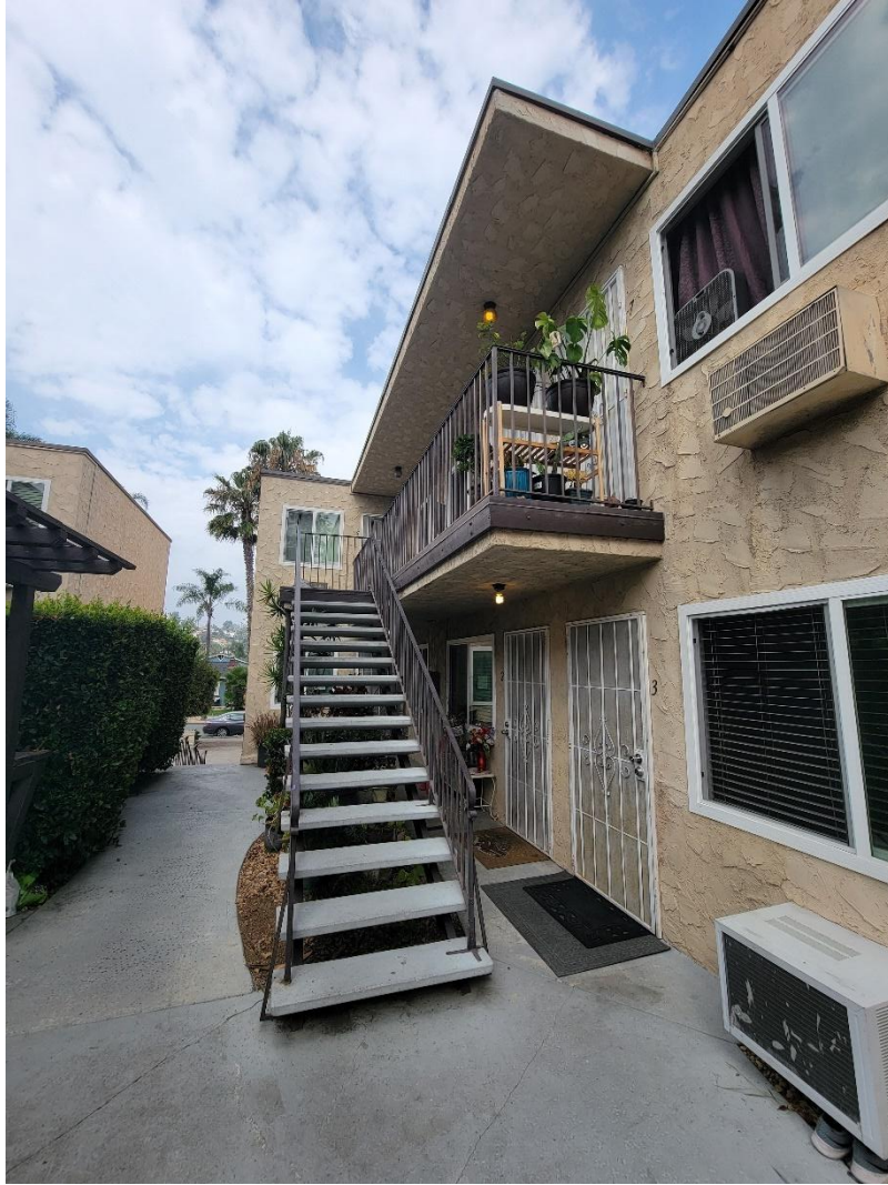
Picture 11: South stair at 4659 3 rd street which all the stair railing and landing railings are wobbly and unsafe.
