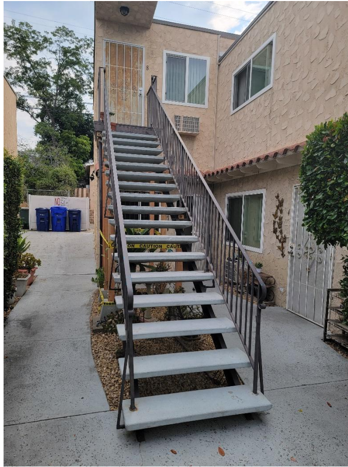
Picture 19: North stair at 4653 3 rd street which the left (west) stair railings is wobbly and unsafe.
