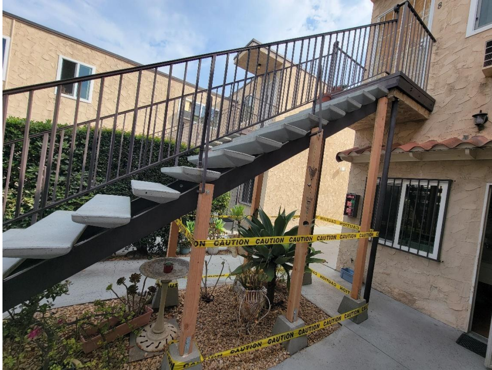
Picture 20: View of north stair at 4653 3 rd street which has been temporarily shored.
