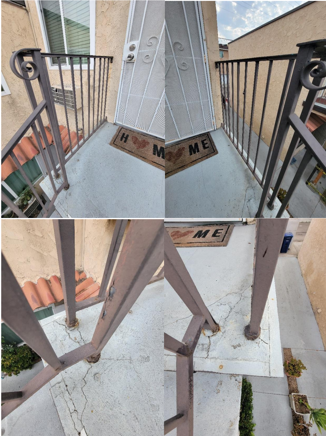
Picture 6: Non-standard post anchorage to the cracked concrete topping on landing.
