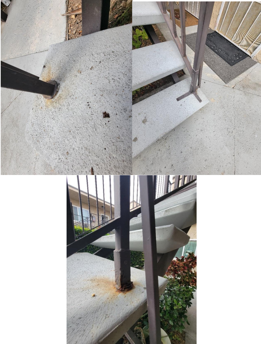
Picture 14: Different non-standard post anchorage to the concrete treads and steel stringer
