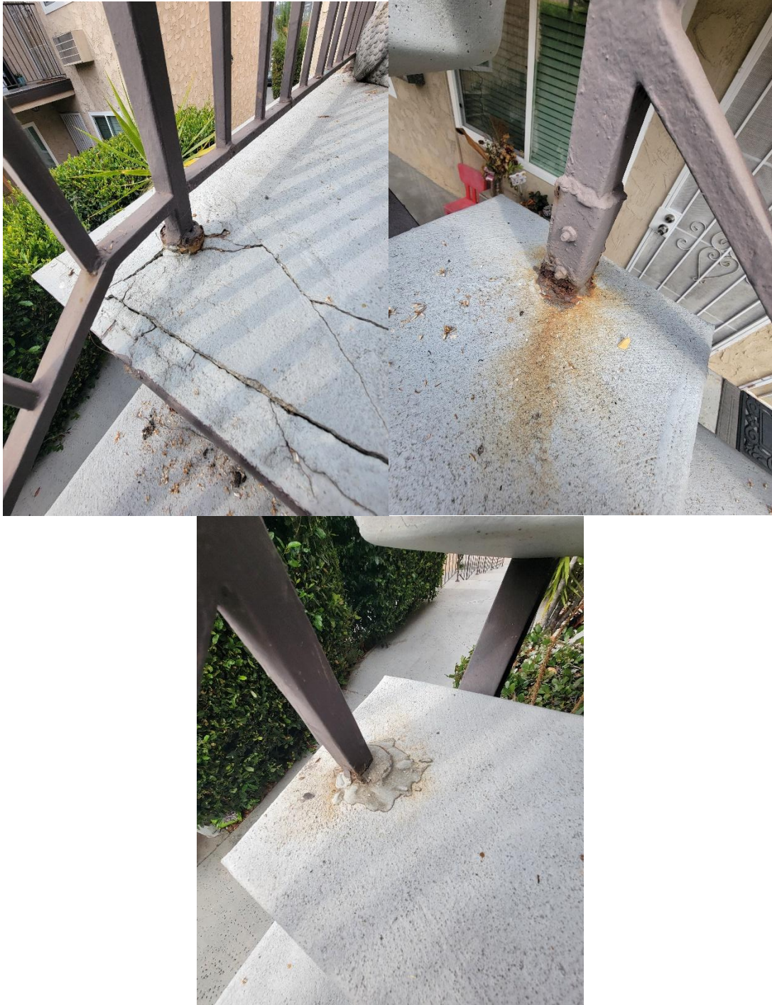
Picture 18: View of stair and landing railing posts anchorage showing corroded post base post and anchorage to the cracked concrete topping which the railing is wobbly and unsafe
