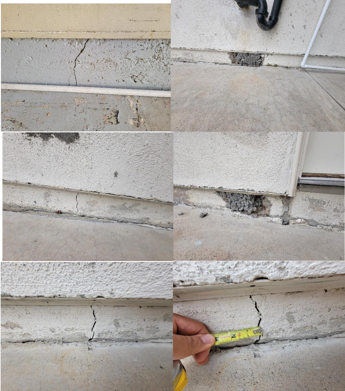
Picture 12: Hairline cracks on concrete stem wall on multiple instances on the garage north wall, and along east side of the garage and the house
