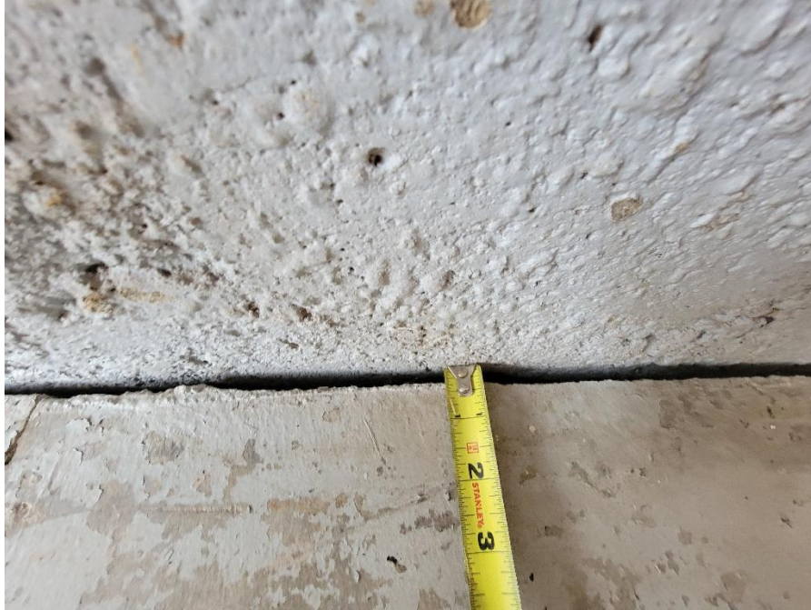
Picture 13: A gap between the garage slab on grade and the concrete stem wall measured to be approximately 3/8"
