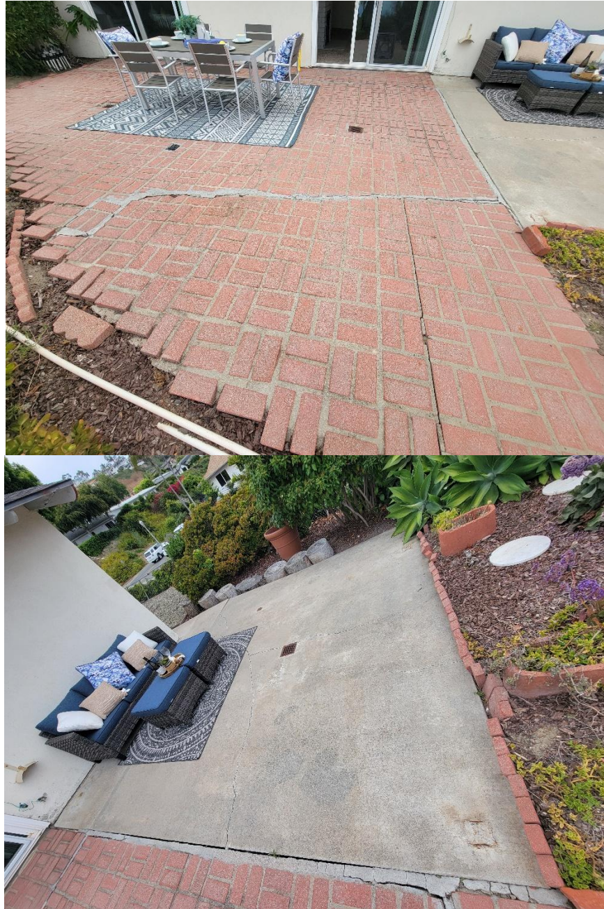
Picture 18: Structural cracks on the backyard paving and concrete slab on grade
