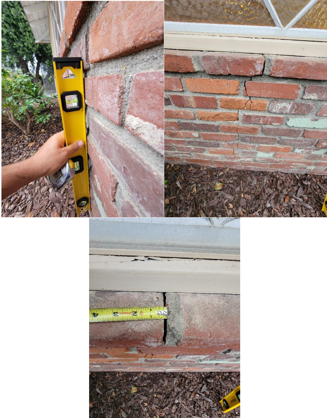
Picture 11: Multiple cracks on brick wall on the garage north wall
