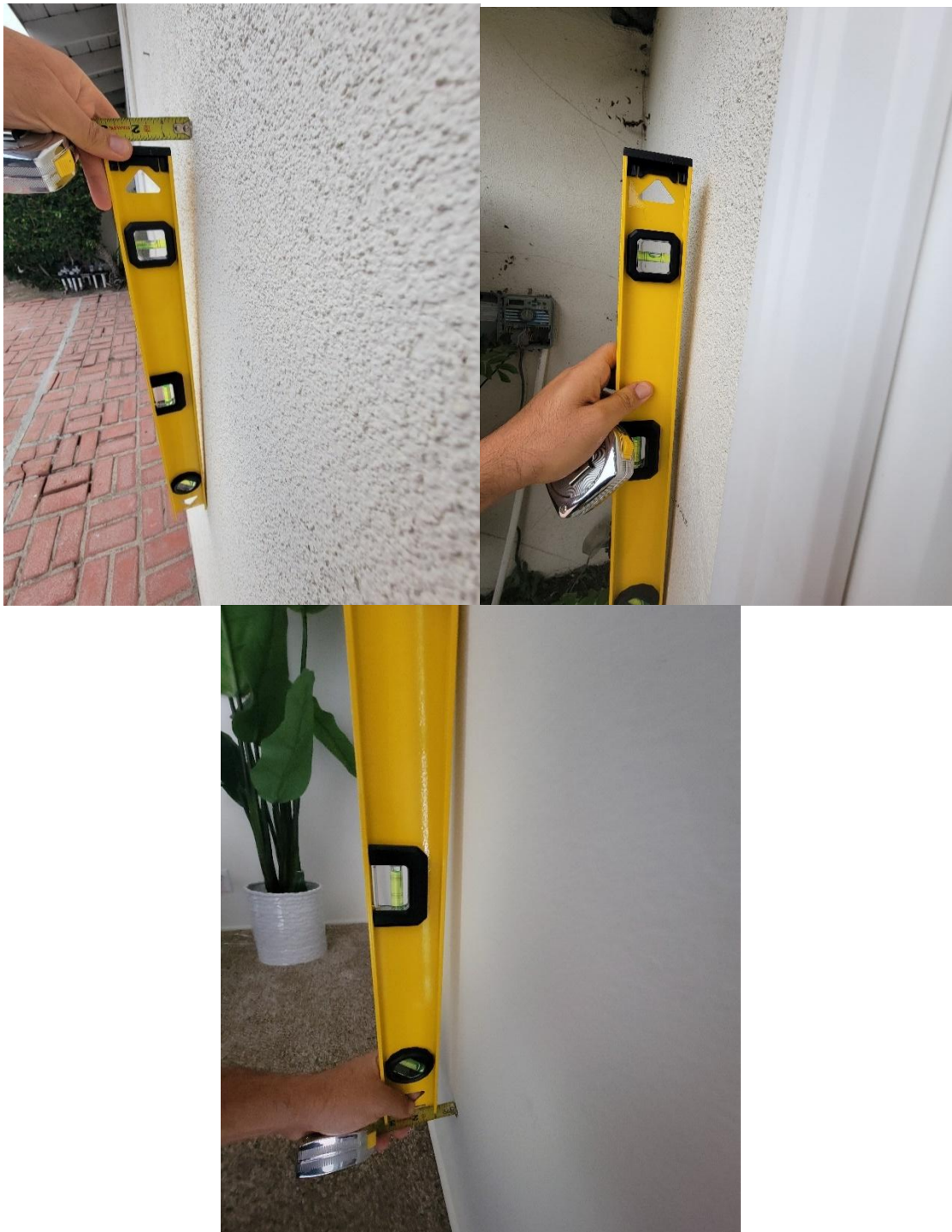
Picture 20: House south wall is not vertically aligned “plumb”, exhibiting a tilt of approximately 2.5 degrees towards the north.
