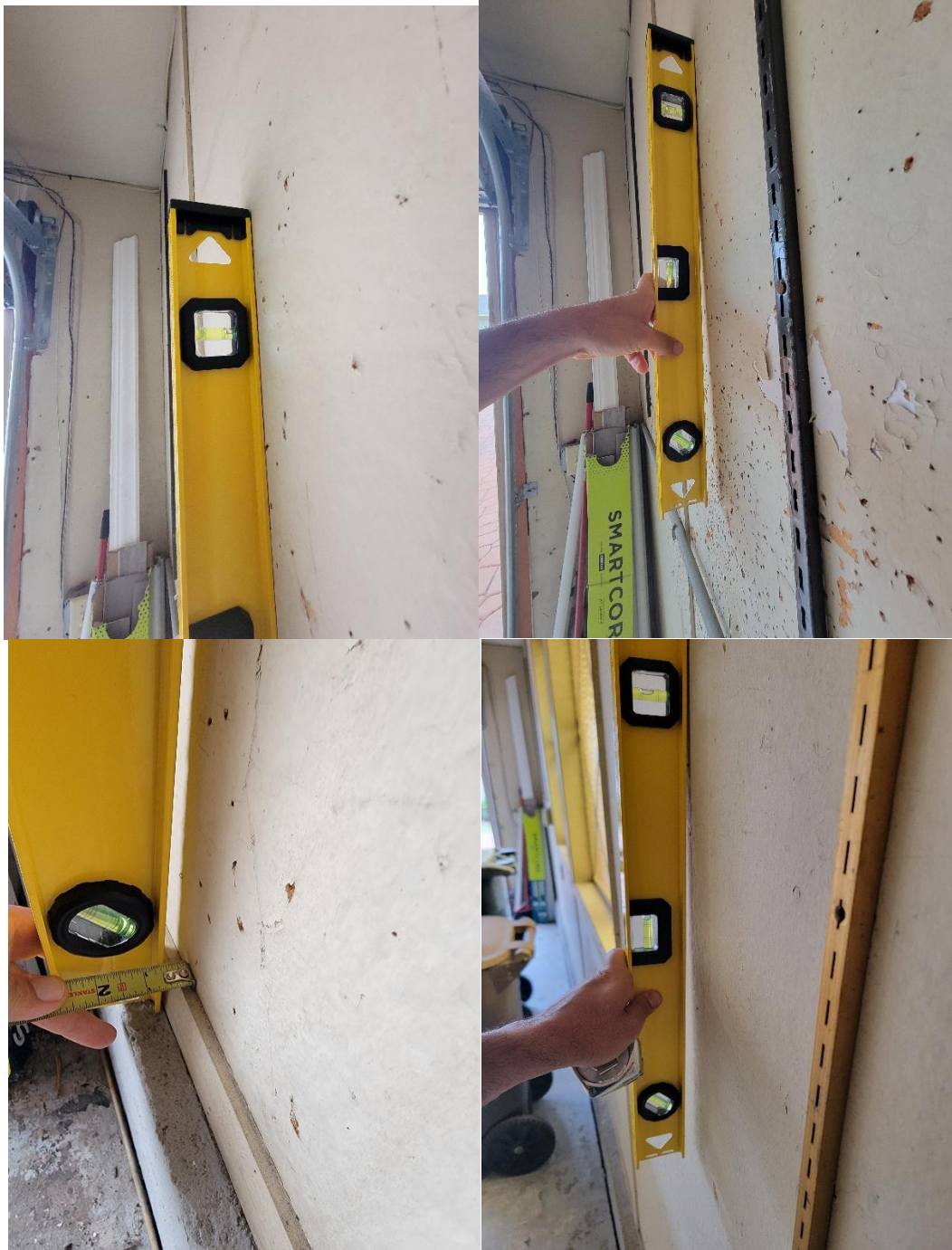
Picture 14: Garage north wall is not vertically aligned “plumb”, exhibiting a tilt of approximately 1.5 degrees towards the south.
