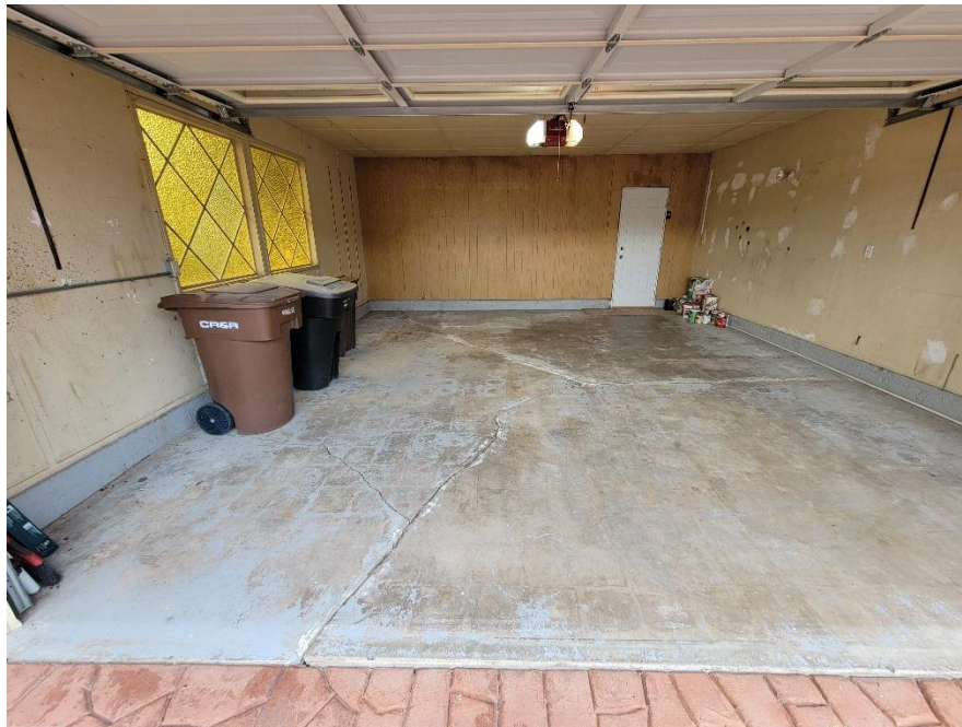
Picture 15: Exterior vertical, and diagonal cracks on stucco specially near the openings and corners
