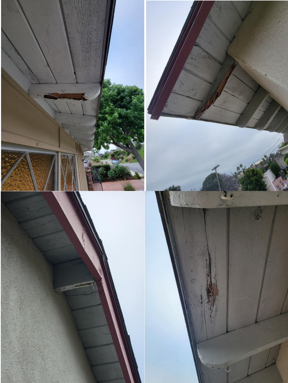
Picture 10: Dry rotted wood elements on multiple locations
