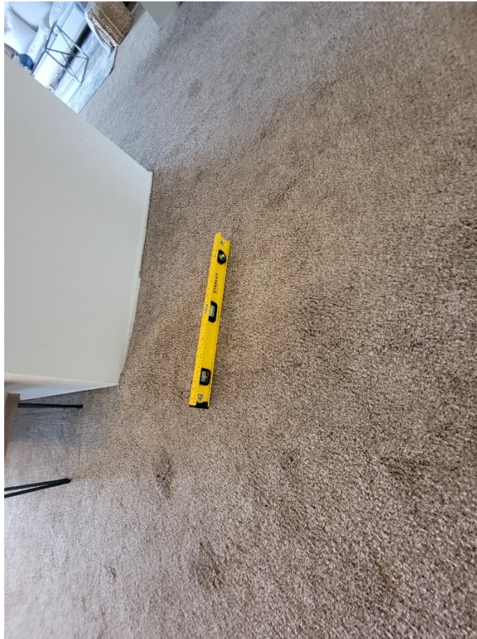
Picture 24: House concrete slab on grade is not horizontally aligned or flat on many locations potentially due to slab on grade cracks, settlement, or slab lift due to potential expansive soil
