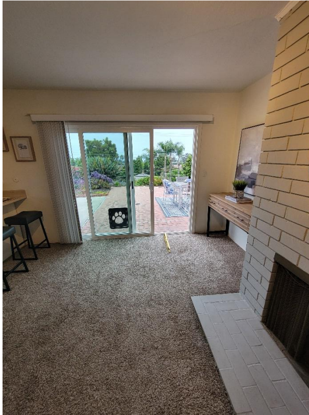
Picture 21: House south wall is not vertically aligned “plumb”, exhibiting a tilt of approximately 2.5 degrees towards the north.
