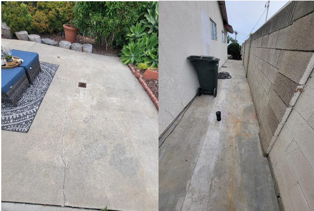
Picture 19: Structural cracks on side yard and backyard paving and concrete slab on grade
